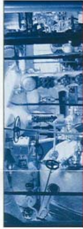
Fire Room on USS The Sullivans
